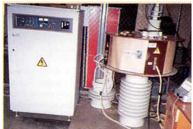
Fig.7. 20 kW, 1 kHz resonant electric power transmission system
